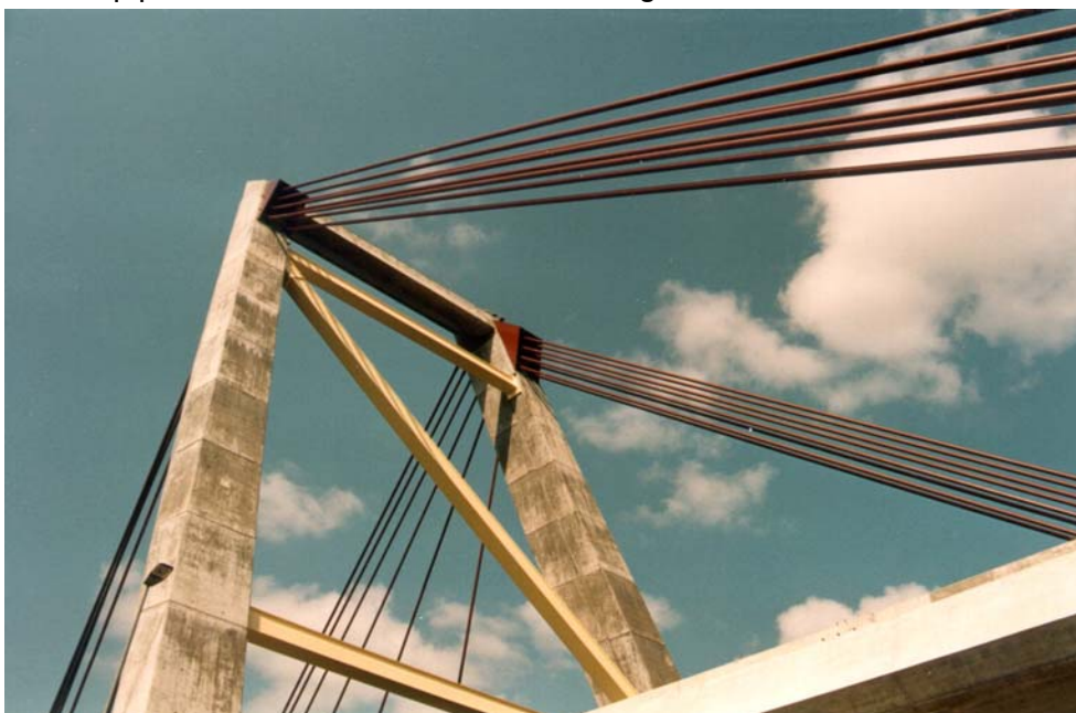
NOFX pipe red-brown on Schaffhausen Bridge, Switzerland
