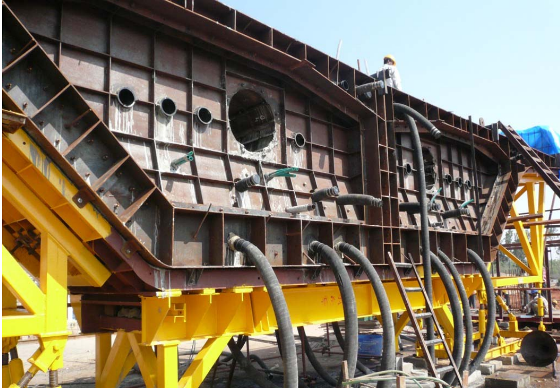
IP 4 S PE Duct on precast segments for Bangalore Elevated Expressway, India
