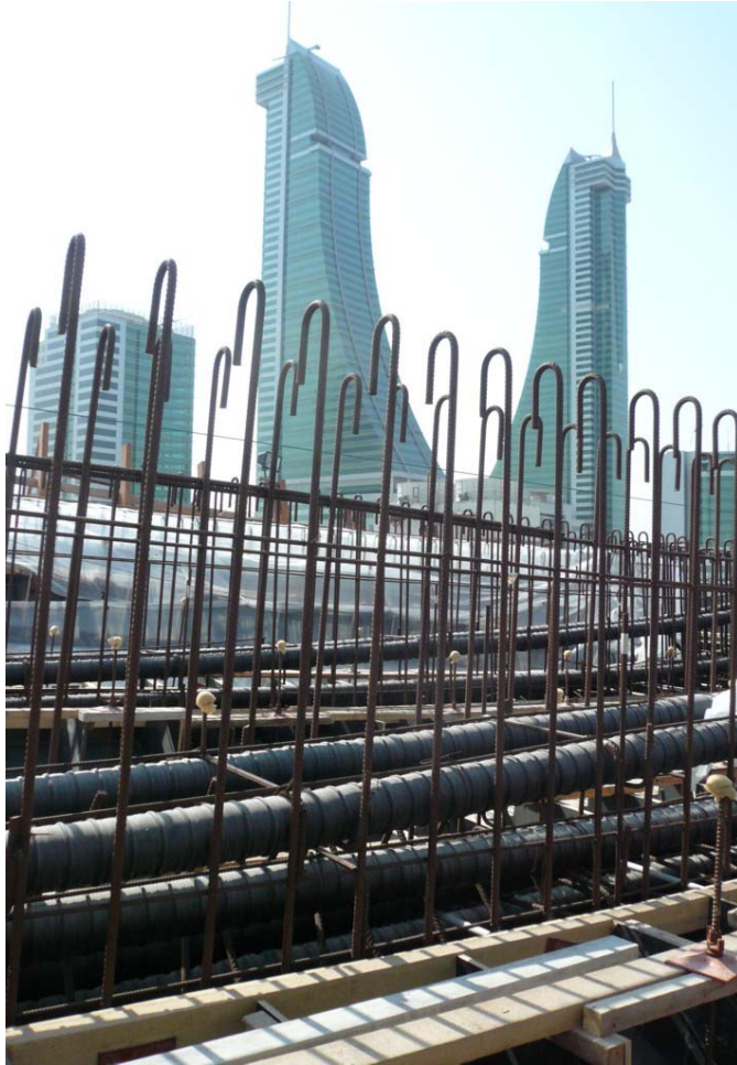
IP 4 M PE Duct on Financial Harbour Bridge, Manama - Bahrain
